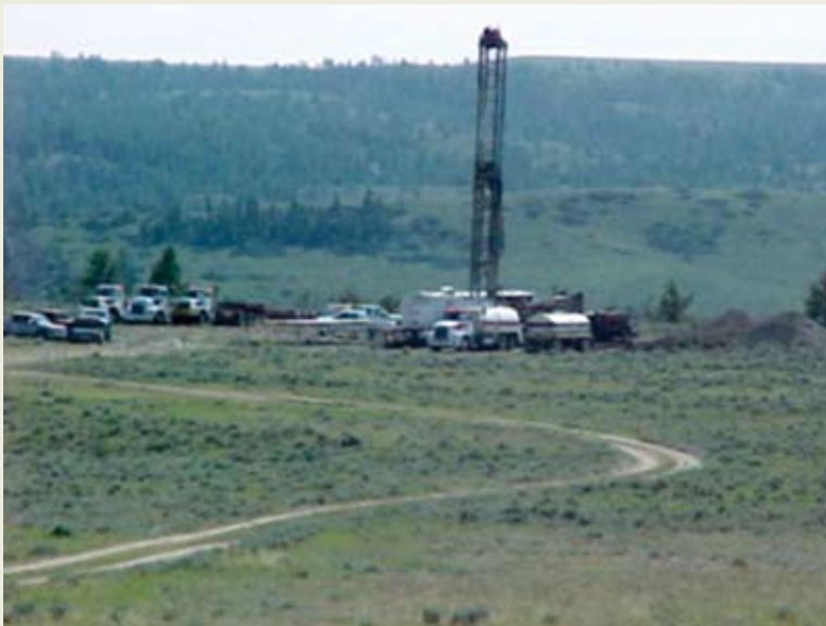
A minimum disturbance, primitive, two-track road winds its way to a drilling operation. To further reduce disturbance, most of the well location has not been stripped of vegetation or topsoil.
